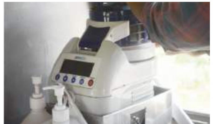
Emvolio installed inside Mobile Health Unit
